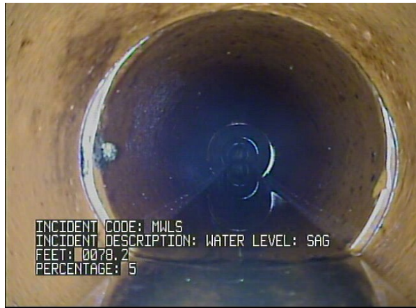
Figure 5 Sag in Pipe Segment MH 030 to MH 029
