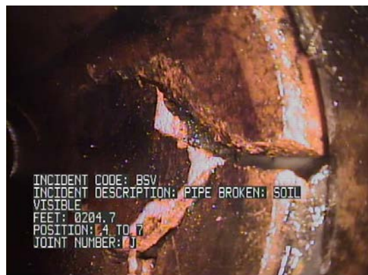
Figure 1 Broken Pipe in Segment MH 033 to MH 032
