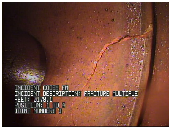
Figure 2 Fractured Pipe in Segment MH 018 to MH 005
