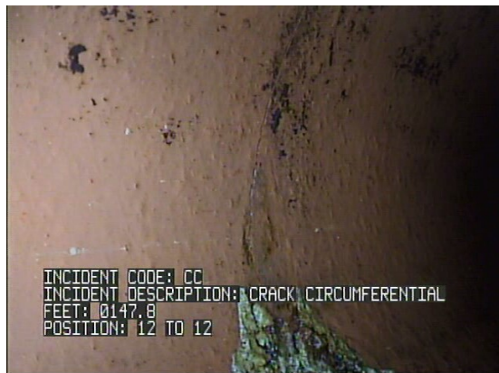
Figure 3 Cracked Pipe in Segment MH 53 to MH 52
