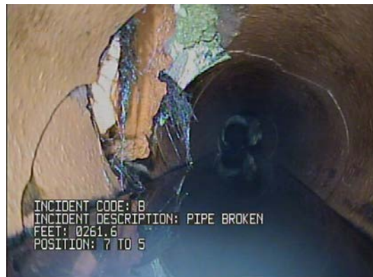
Figure 1 Broken Pipe in Segment MH 54 to MH 53
