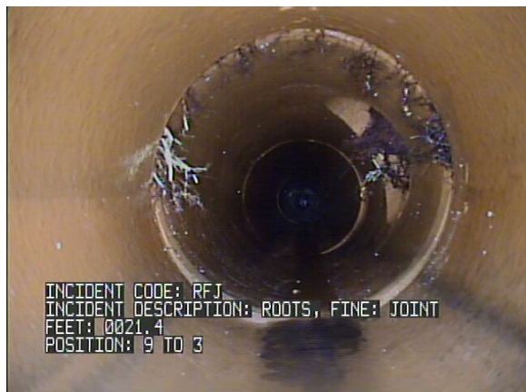
Figure 6 Root Intrusion in Segment MH 66 to MH 65
