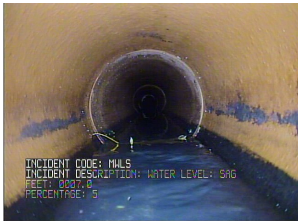
Figure 5 Sag in Pipe Segment MH 49 to MH 48
